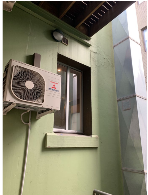
22 Detail view of rear elevation of 15-17 Hunter Street showing original window opening, recently replaced deck/balcony above
